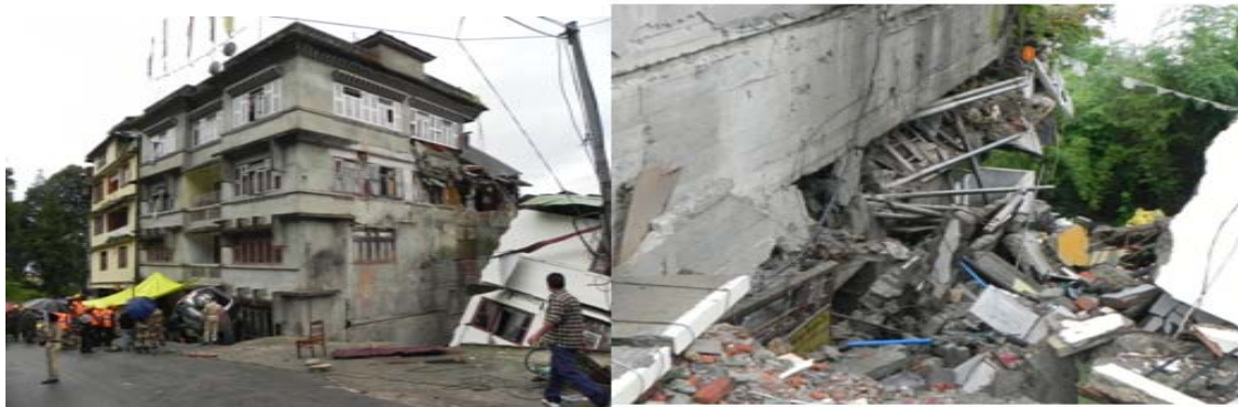
Figure 2 Failure at sixth (road level) storey of a ten storey hill building during Sikkim earthquake of September 18, 2011
